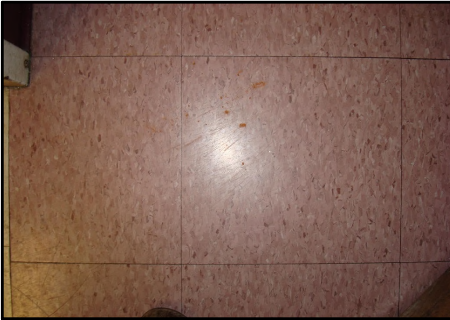
Photograph No. 16 View of floor tile located in the toddler and pre-school rooms.
